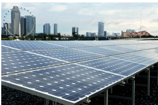
Picture courtesy of PUB The largest Solar Park in Singapore at the Marina Barrage covers an area of 1,200sq m. The 405 solar panels generate electricity used for indoor lighting and power points in the Marina Barrage.
